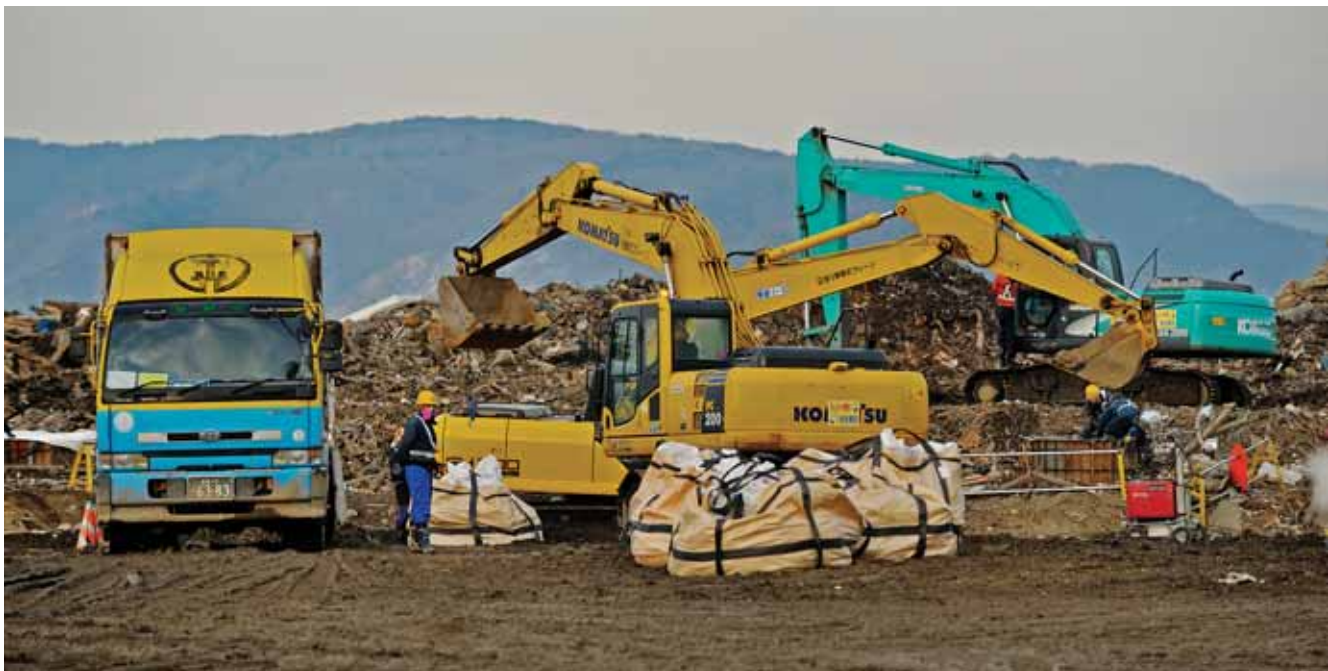
The disaster generated an unprecedented volume of debris which will take several years to clean up
