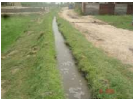
Figure 23.2 Pond waste water outgoing open drain
